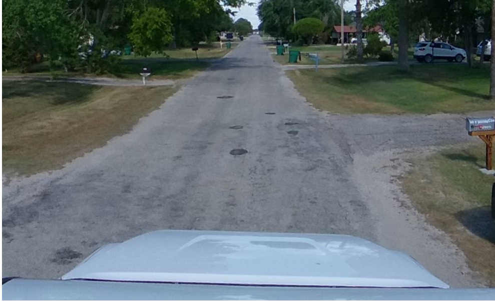
Bowl shaped holes caused by weakness in pavement and progressive deterioration.
