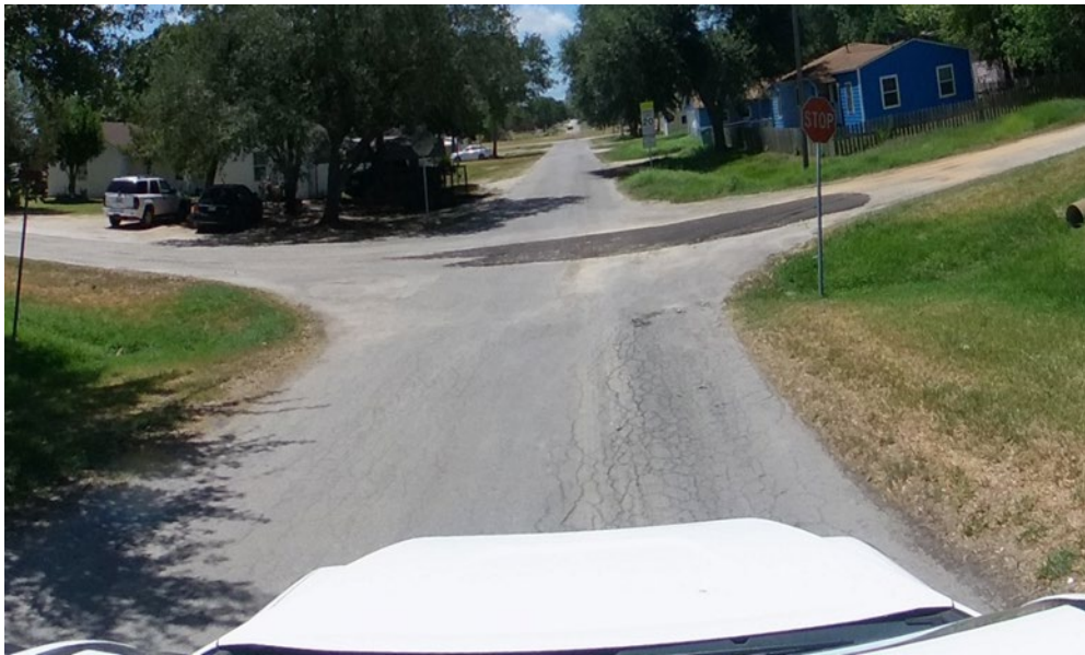
Series of cracks in pavement usually caused by unstable subgrade or movement in the ground.
